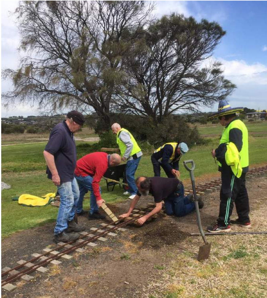
A happy gang of PBMR "fettlers" doing track repairs along the line. (Pic : Brian Coleman) (Left to right - Alistair Blues, Brian Parkinson, Don Gill, Harm Jager, Ronnie Frank, Robert Freeman)
